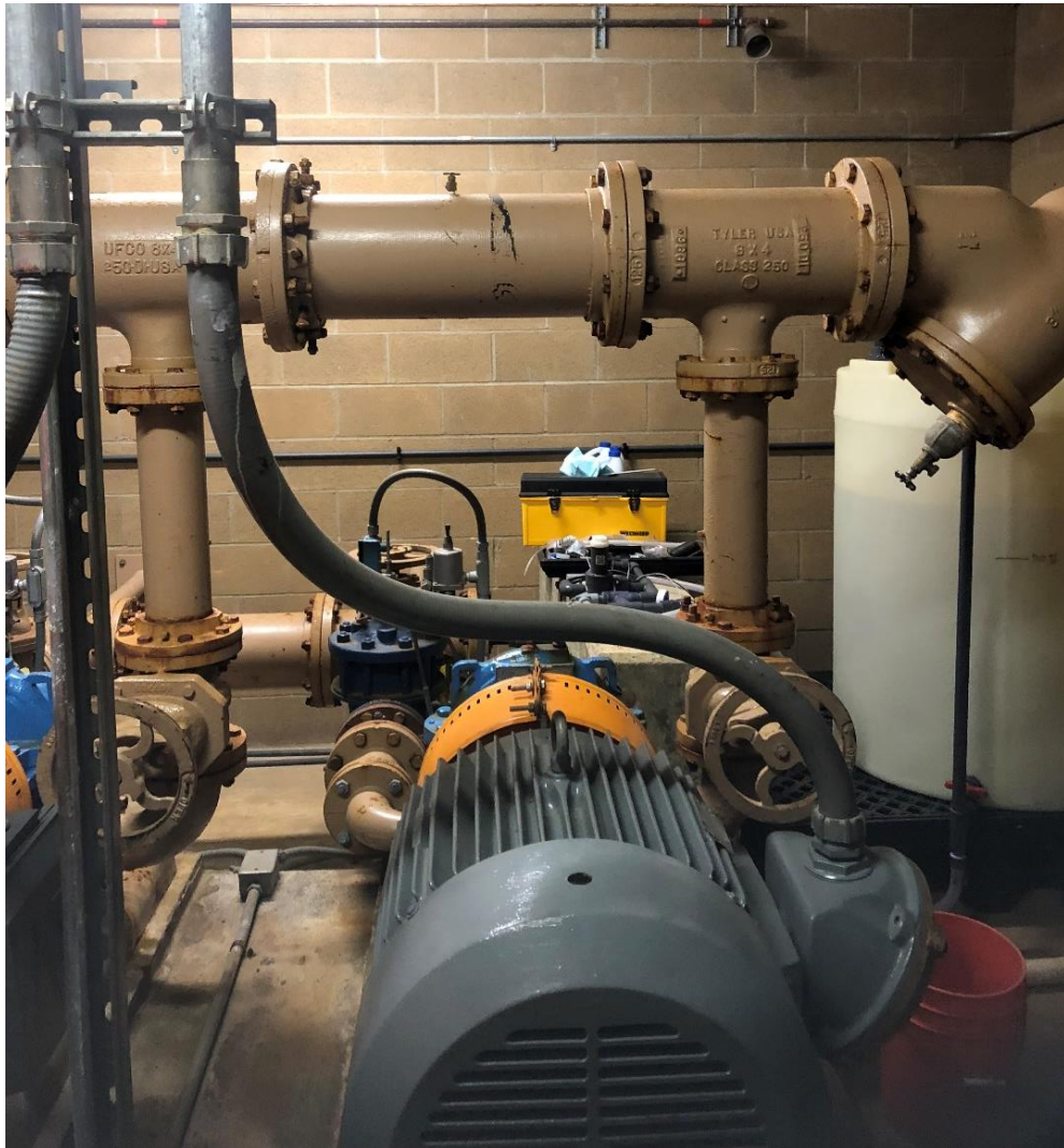
North Bank Pump Station
