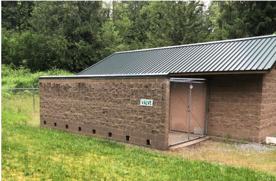
North Bank BPS (Outside)
