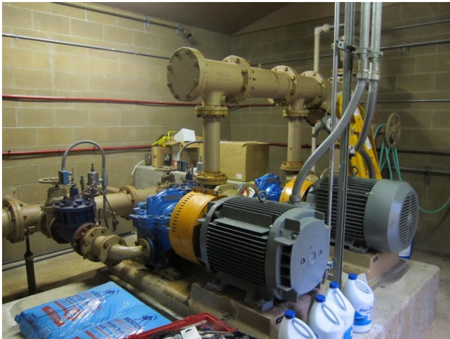
North Bank BPS (Inside)
